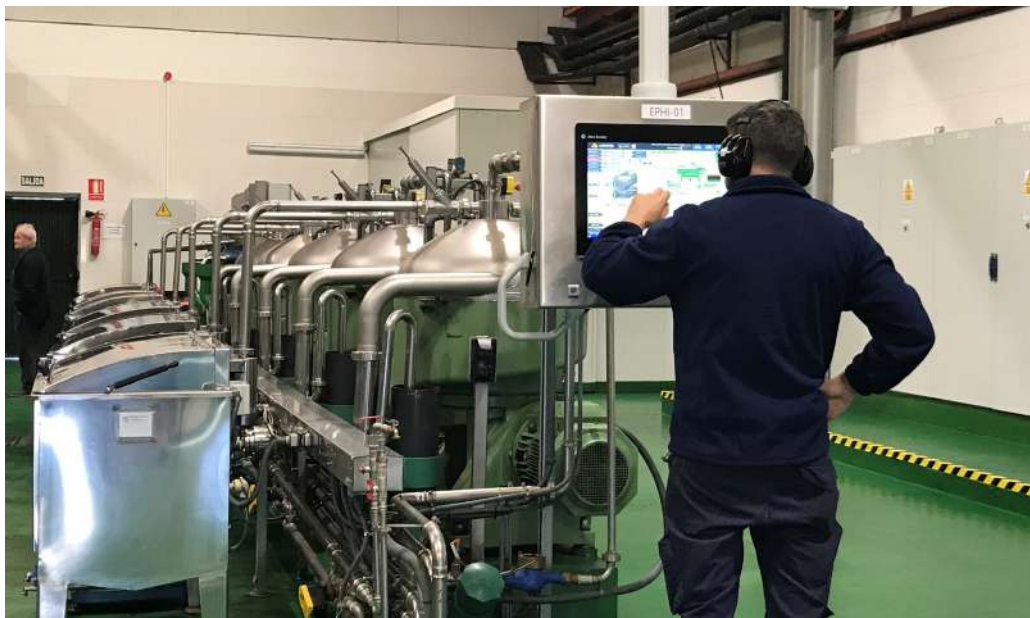
Local operation system at the Extraction Room next to the Vertical Centrifuges, which offer the same integral visualization and operation benefits as the control room at the shop floor
